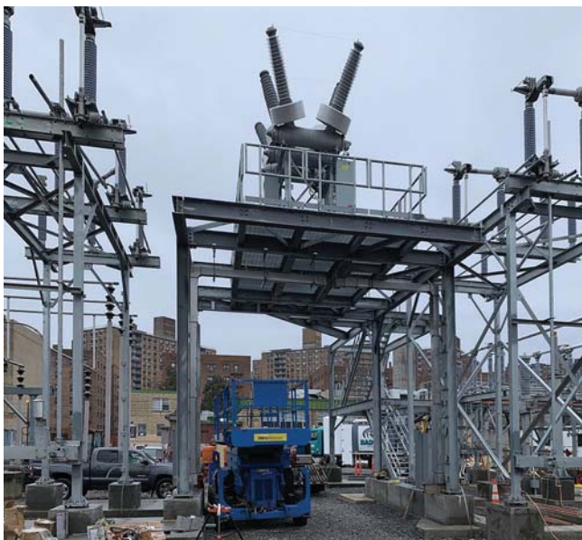
The Rainey Substation from the ground up. In May 2023, Con Edison crews completed a 6-mile (9.7-km) line that connects two substations in Queens. Photo courtesy of Con Edison.
