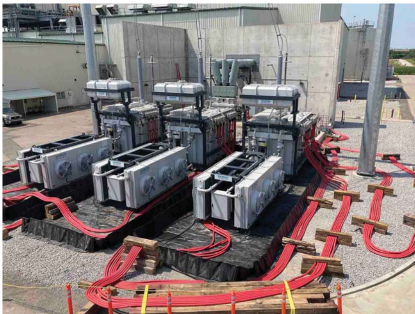
GSU lease transformer. Courtesy of Siemens Energy.
