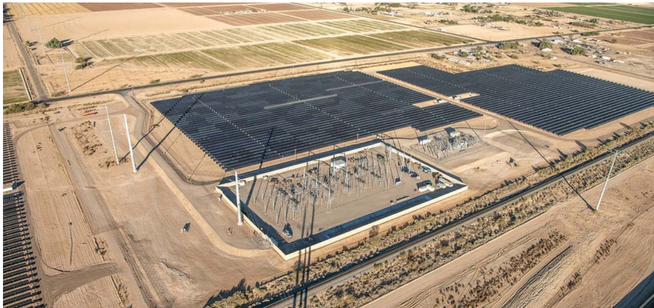
SRP announced an additional 100 MW, 400 MWh of battery storage to be added to the existing Saint Solar facility in Coolidge, AZ. Photo by Salt River Project.
