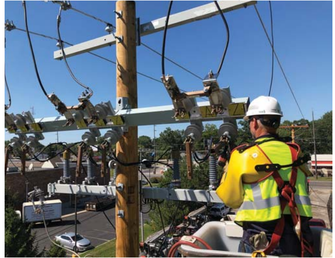
Visibility and management of the overall network extends beyond the control room. Line workers can see what's happening with the app. Photo by FirstEnergy.
