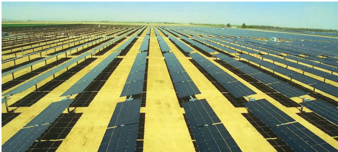
The Pinal Central Solar Energy Center became operational in 2018 and consists of a 10-MW battery system powered by 20 MW of solar generation. Photo by Salt River Project.
