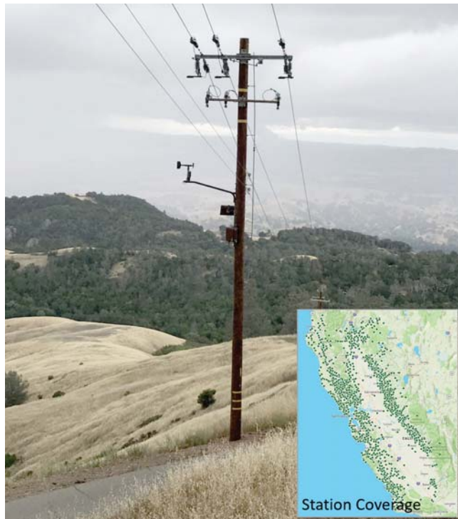
PG&E weather station installed on Mt. Diablo in the East Bay Area. Inset map shows PG&E's weather station coverage of ~1500 weather stations.
