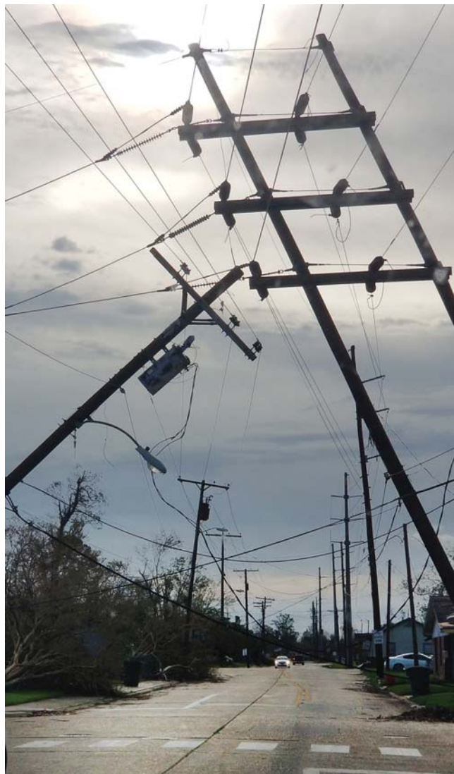
Wood pole storm damage image taken by an Osmose employee. Photo by Osmose.
