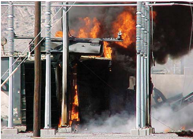
Burning transformer. Photo by Gene Wolf.
