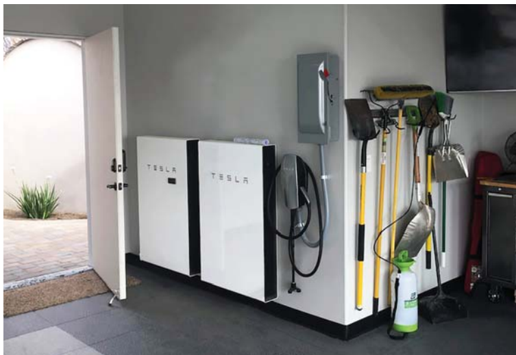
Swell Energy, California Install. Photo by Swell Energy/SMUD
