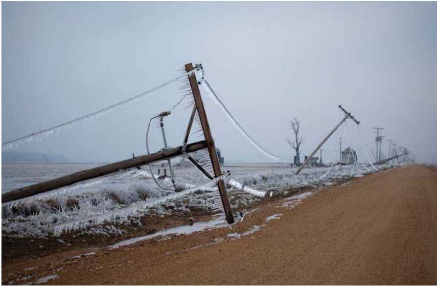
Storms and severe weather are the No. 1 cause of downed power lines and power outages. Photo by iStock.
