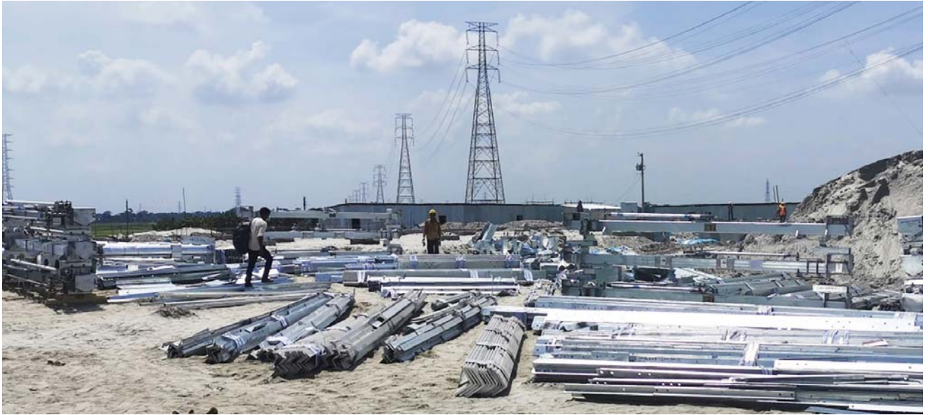
View of 400-kV tower from Gopalganj substation.
