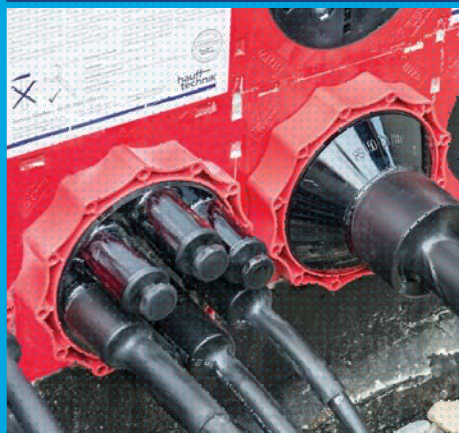
System covers connect to cables and conduits
