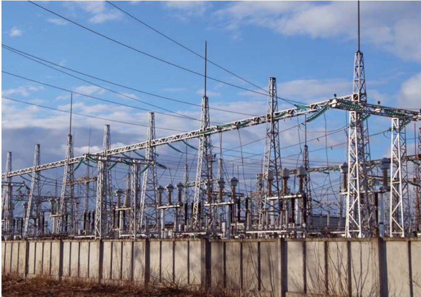
A high voltage substation in Texas. Because of the storm knocking power plants offline, ERCOT reported that the Texas power grid was minutes or seconds away from collapse before partial shutdowns were ordered. Photo by Getty Images
