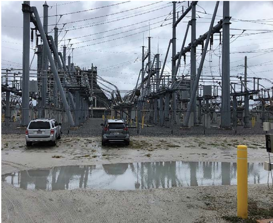
Upgraded and hardened substation key part of new, reimagined microgrid. Photo courtesy of the authors.
