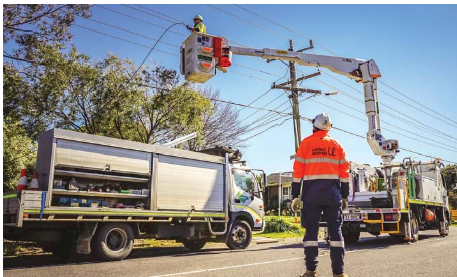
A large portion of United Energy's network is overhead and exposed to a variety of potential sources of damage. Through the use of digital monitoring systems, however, United can detect and receive alerts about irregularities on the network caused by such incidents. Photo by United Energy.
