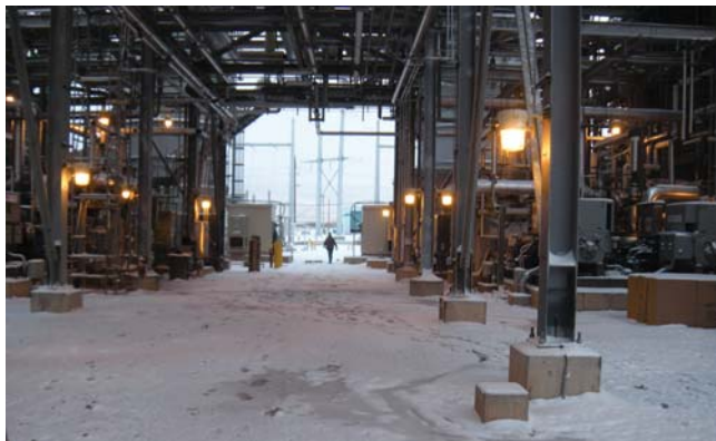
Extreme cold hits one of El Paso Electric's power generating units during the 2011 winter storm. The utility says this storm led it to harden its assets against future freezes. Photo by El Paso Electric
