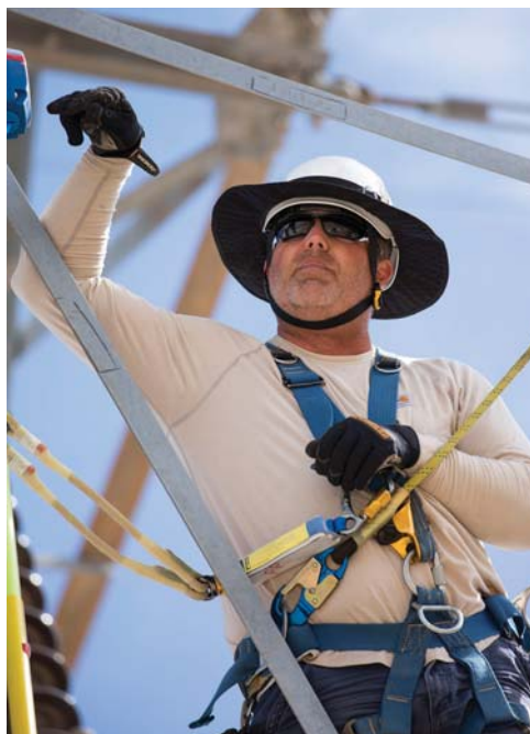
David Katich of Western Area Power Administration (WAPA) and IBEW 769 performs aerial patrols.
