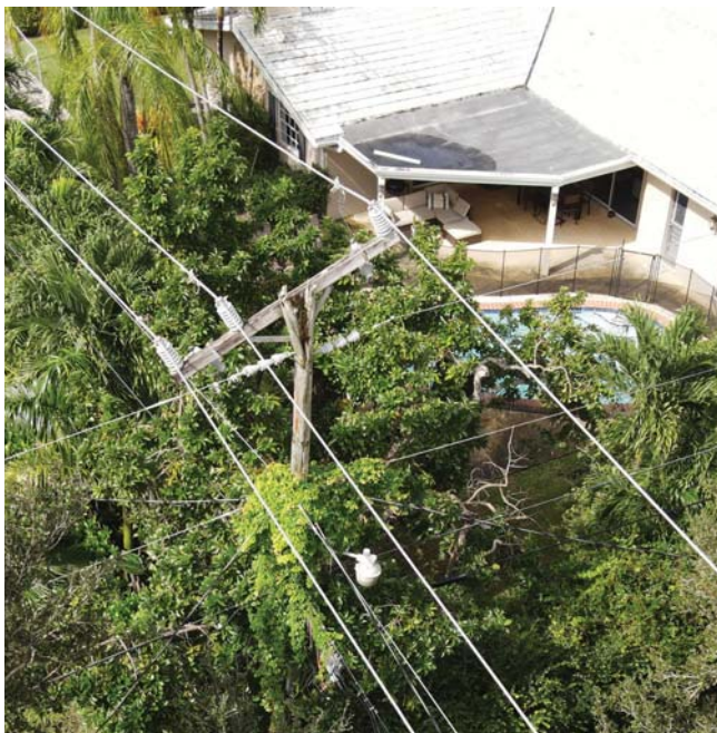
Through the use of drones and various sensors, BHI Energy can scan any areas of interest, like the broken pole shown above.
