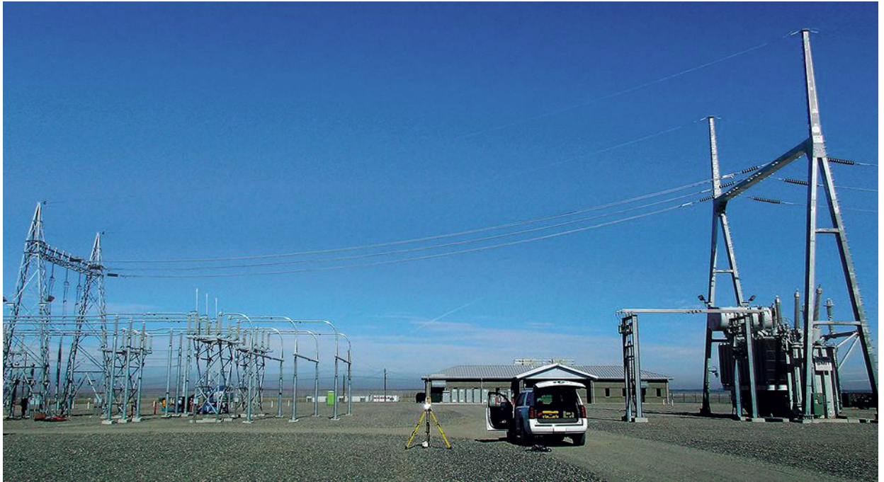
After the inspection, linemen were able to correct the sag. HiLine has discovered problems with transmission line sag nationwide.
