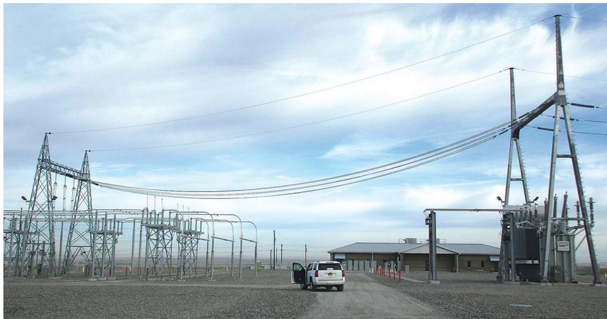
The line crew believed that this conductor was at engineer design sag, but an inspection found that it was not sagged properly.
