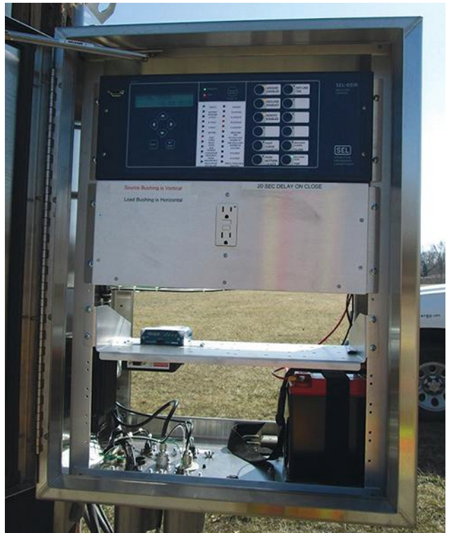
To accommodate automated switching in the field, the SmartStar distribution automation system uses the SEL-651R advanced recloser control, the SEL-2401 satellite-synchronized clock and Sierra Wireless 3G cellular modems.
