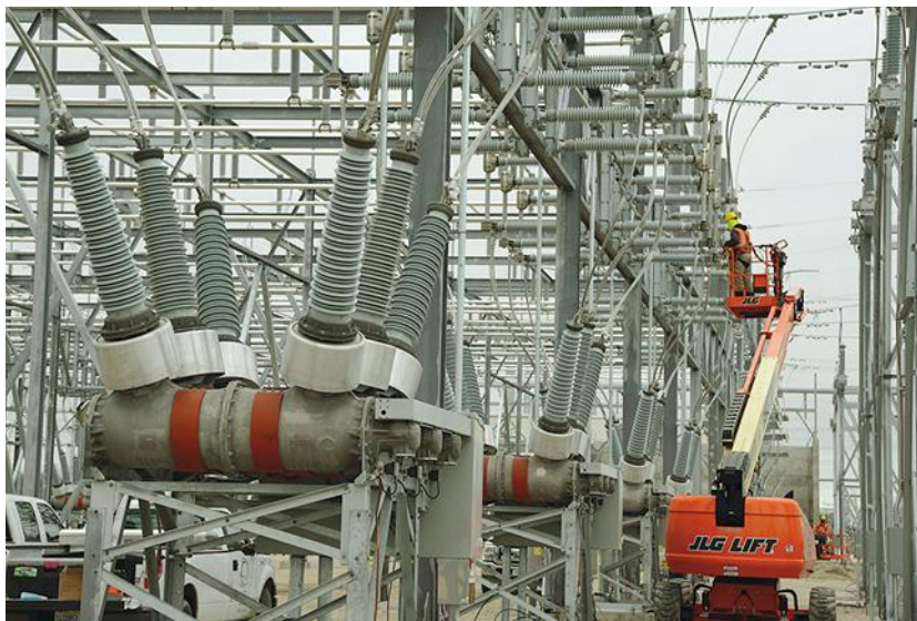
Substation equipment is inspected, and the results are used as one of many inputs in the derivation of equipment health indices.
