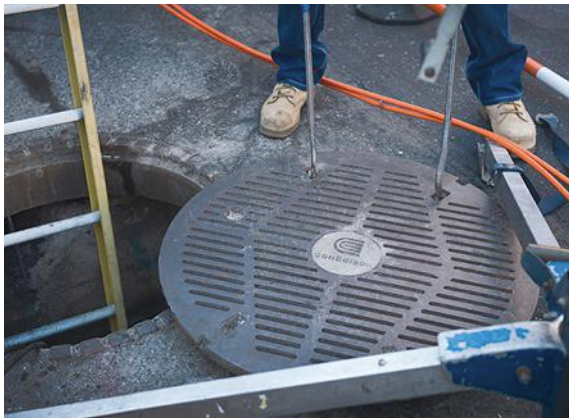
By replacing solid manhole covers with vented covers, Con Edison has been able to protect its field workforce when working underground.
